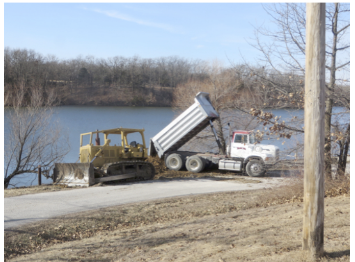
Construction of an earthen fishing pier should improve success of shoreline anglers at Thayer City Lake. This shows the first day of work in constructing the pier.
